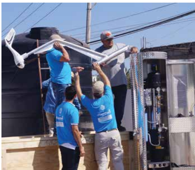
Rotarians from Redwood City, California, USA, assemble a solar-powered water purification system in San Miguel de Allende, Mexico.
